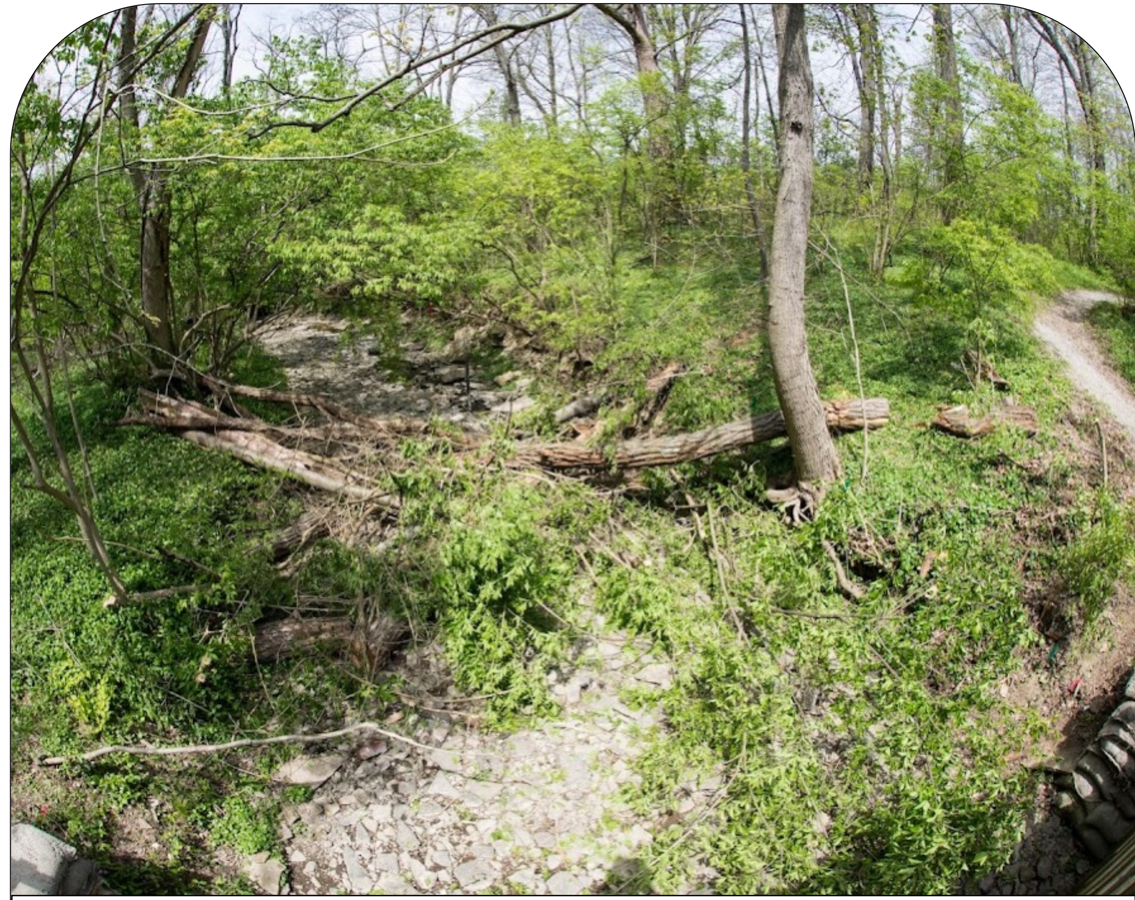
Log jams, like the one pictured above, were installed in Cooper Creek to help slow water velocities, reduce erosion, and create deep pool habitat.
